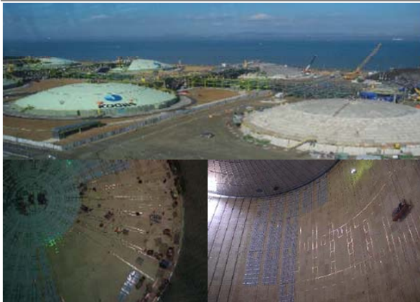
Figure 6. In-ground LNG storage tank
