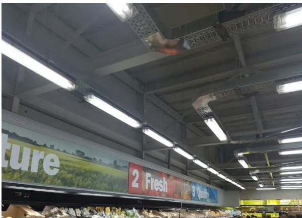
Figure 9. No Brand store: No finishing materials on ceiling
